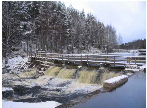
Fig. 2. Part of the dam at the pilot power plant, picture taken 29 th November 2007. The generator pool is on the right (partially visible). As can be seen, the hydrological situation is such that the inflow is greater than the plant's capacity, and the spillage is high.
