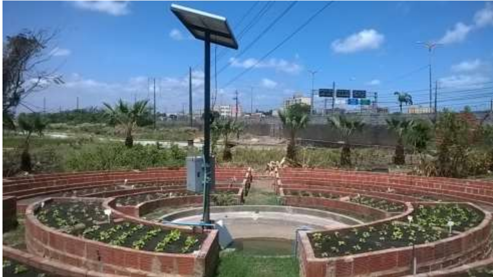
Fig.3. PV powered irrigation system applied to familiar agriculture
