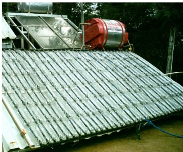
Fig. 3, ASBC installed on Renewable Energy Center of UNESP, Guaratinguetá, SP. Fonte: (Author, 2014)
