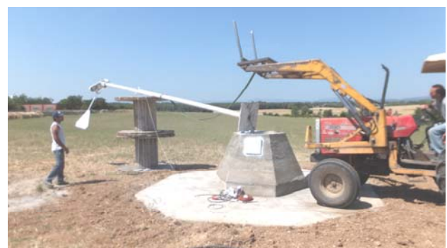
Fig. 5. Small wind turbine installed in a farm located in Ordis
