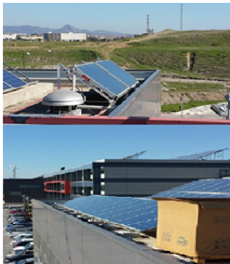
Fig.2. View of the Photovoltaic modules and thermal collectors
