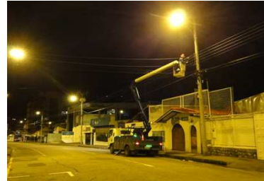
Fig. 3 Supply voltage readings with the device CL3121 on Heroes de Verdeloma Ave. and Eugenio Espejo street.
