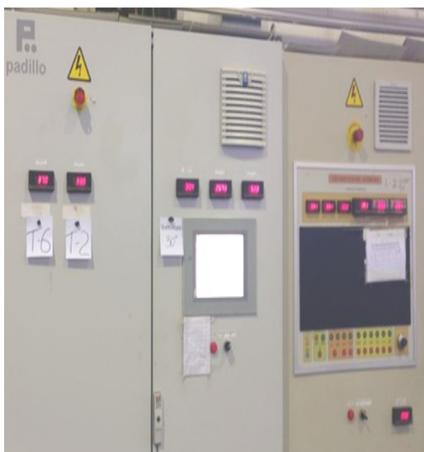
Figure 1. Electrical panels of the oil mill.
