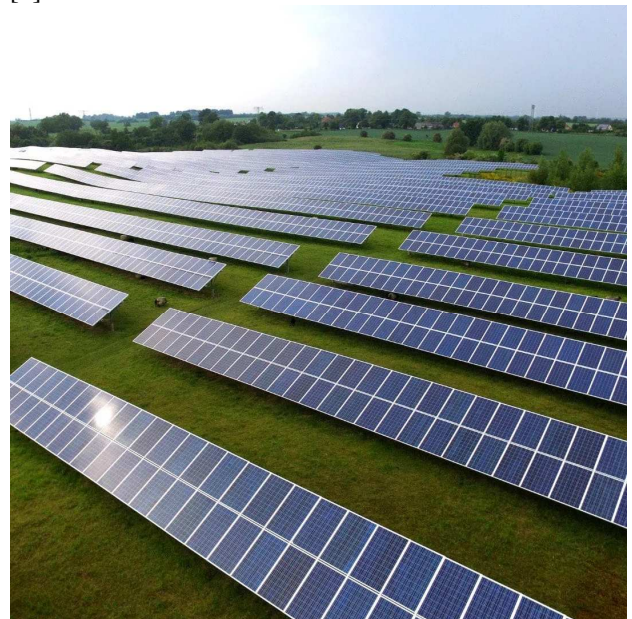
Fig. 2. Large PV plant in the Netherlands
