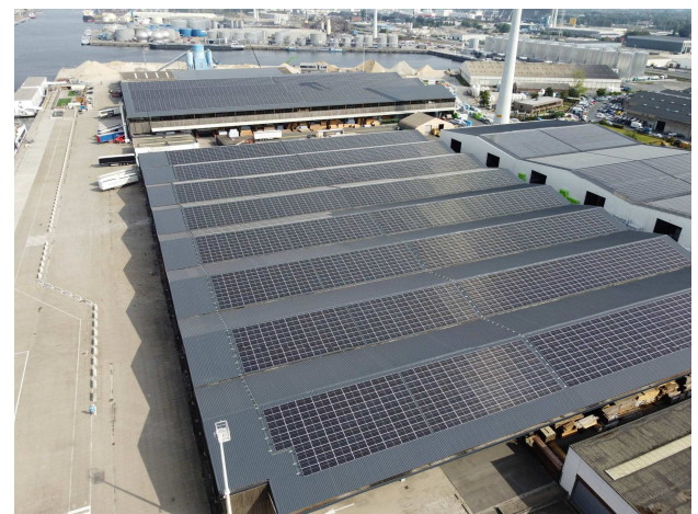
Fig. 13, 1MWp project at Ghent Harbor
