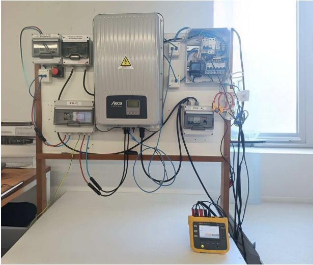
Fig. 2. Board used in the On-Grid system.
