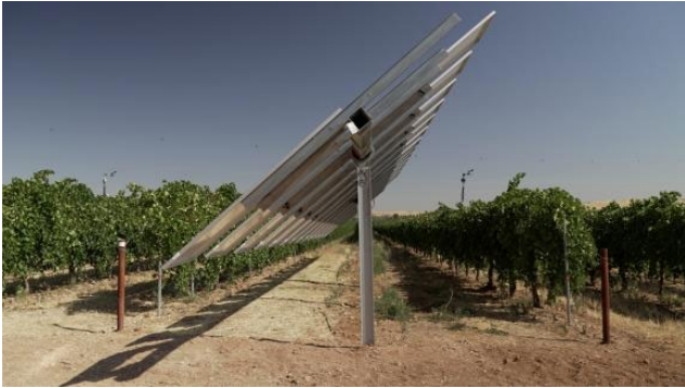
Fig. 5. Installation of smart photovoltaic panels in a vineyard. An example of how renewable energy generation coexists with the rural environment.
