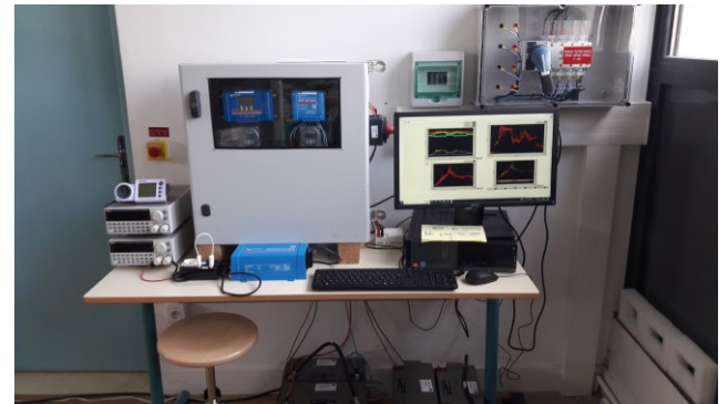
Fig. 4 Photo of the two systems installed in the electrical cabinet. (The batteries are under the table, the stand-alone inverter is on the table with the measurement PC and active loads. The solar panel connections are at the top right.).
