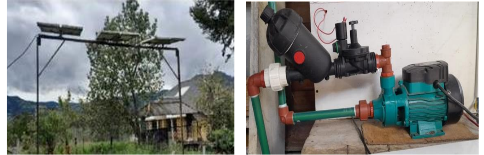
Fig 3, PV structure for agrovoltaic system and hydraulic system
